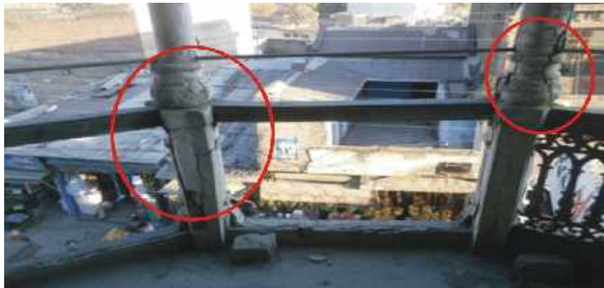
Figure 16 - Major cracks can be seen
