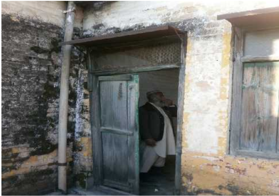
Figure 24 - Black crust on the wall of second floor
