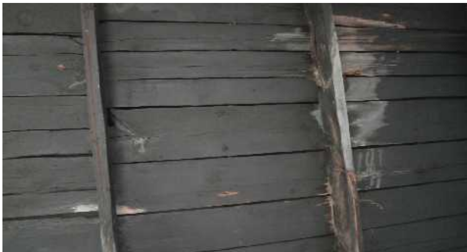
Figure 11 - Smoky black ceiling on second floor
