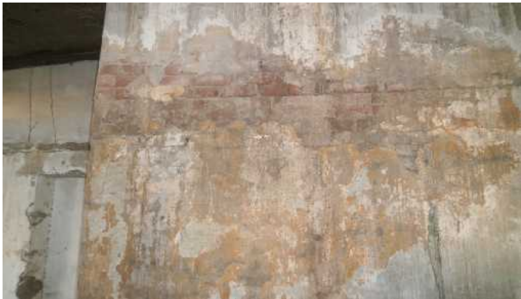
Figure 14 - Brick decay can be seen on second floor
