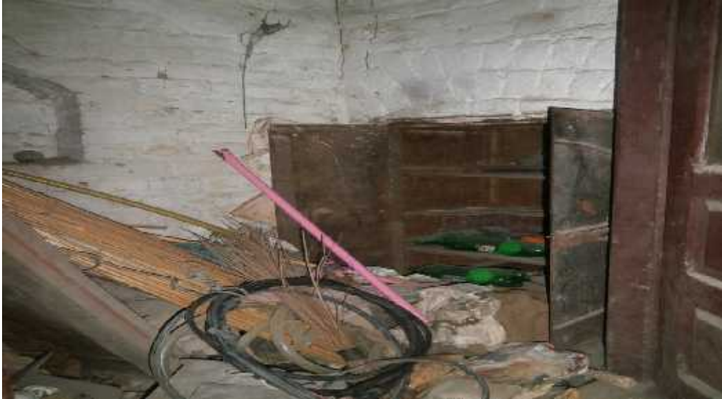
Figure 12 - Waste and garbage on first floor
