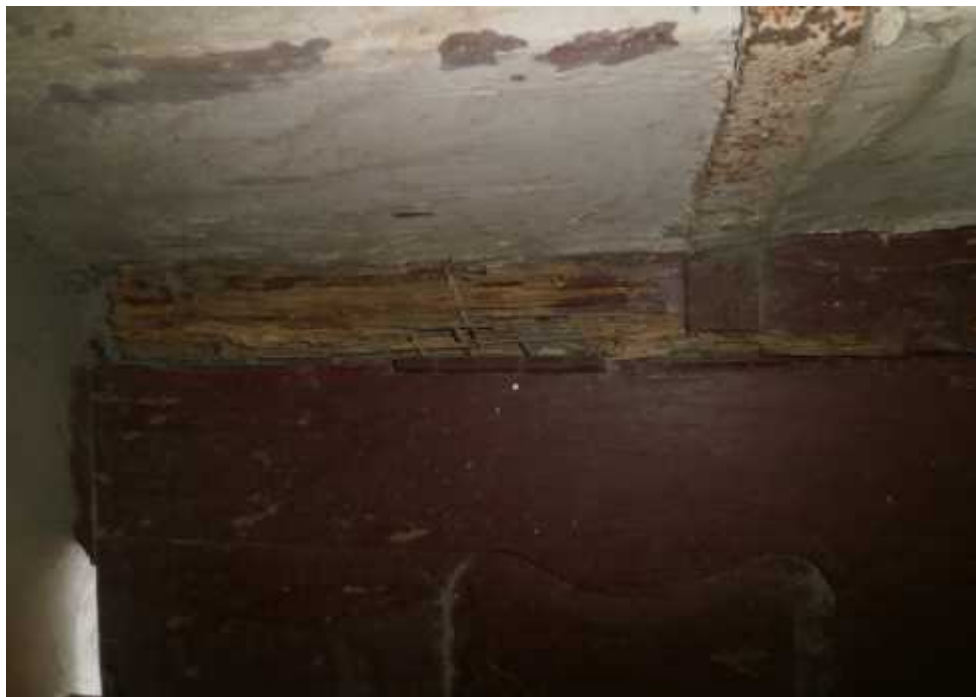
Figure 26 - Termites attack on door of ground floor
