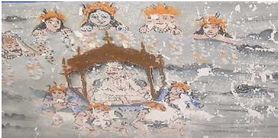
Figure 20- Decayed painting on the ceiling of Gurudwara on ground floor
