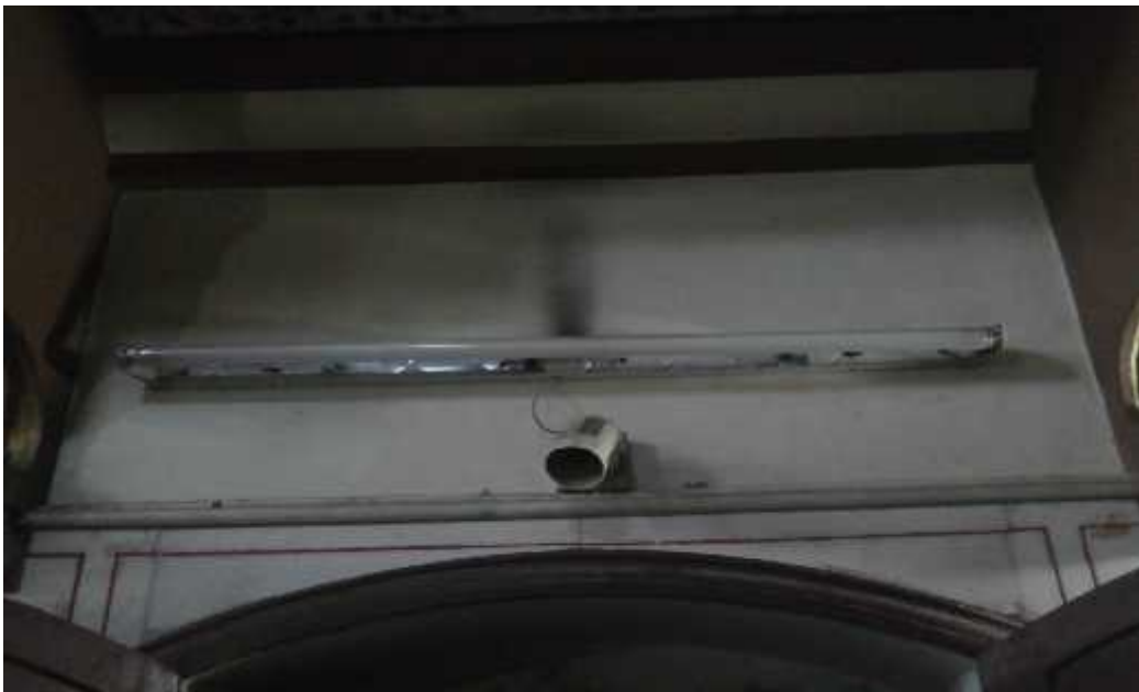
Figure 13 - Black soot caused by the short circuit on the wall of the ground
