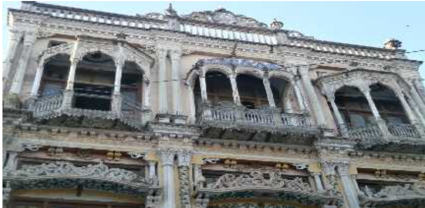
Figure 17 - Stucco decay on facade
