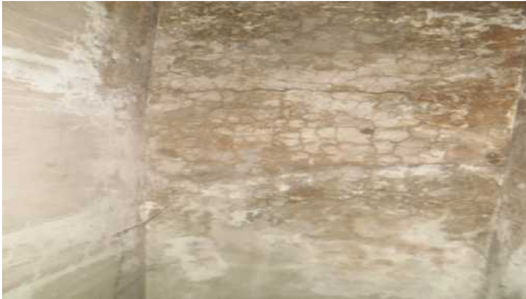
Figure 23 - Stains due to leakage on the ceiling of second floor
