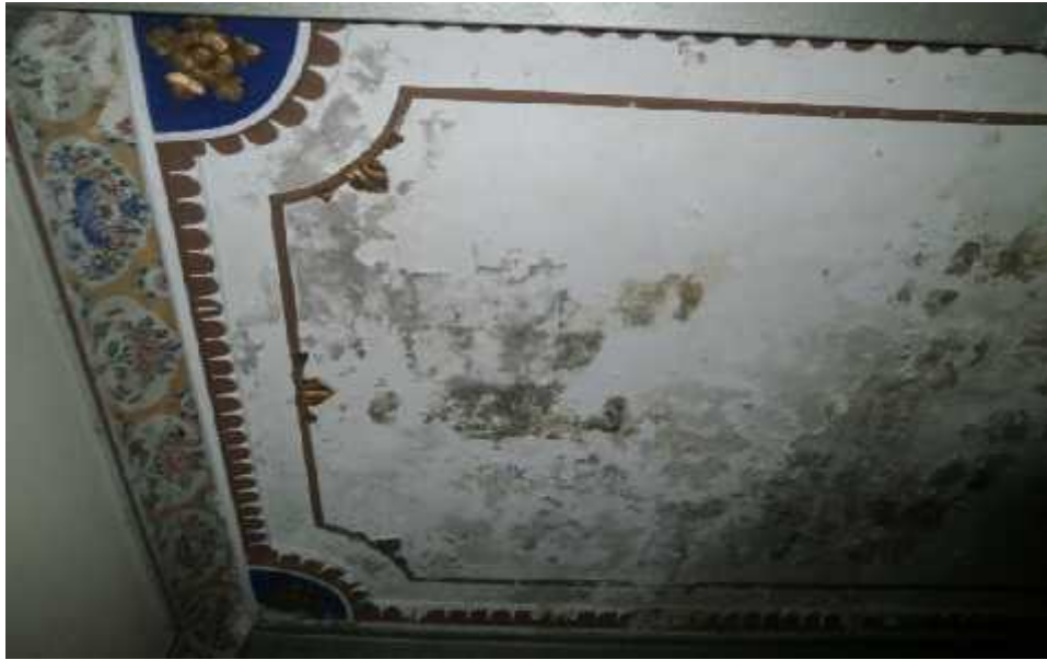
Figure 19 - Plaster decay can be seen
