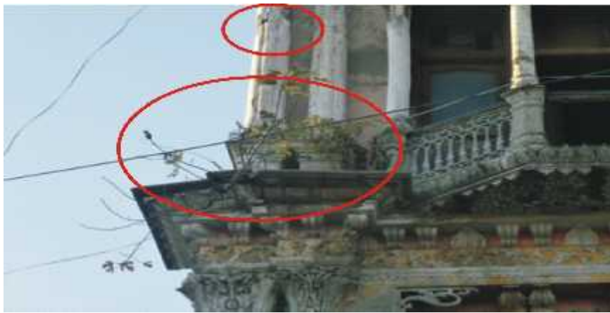
Figure 18 - Cracks and vegetation growth
