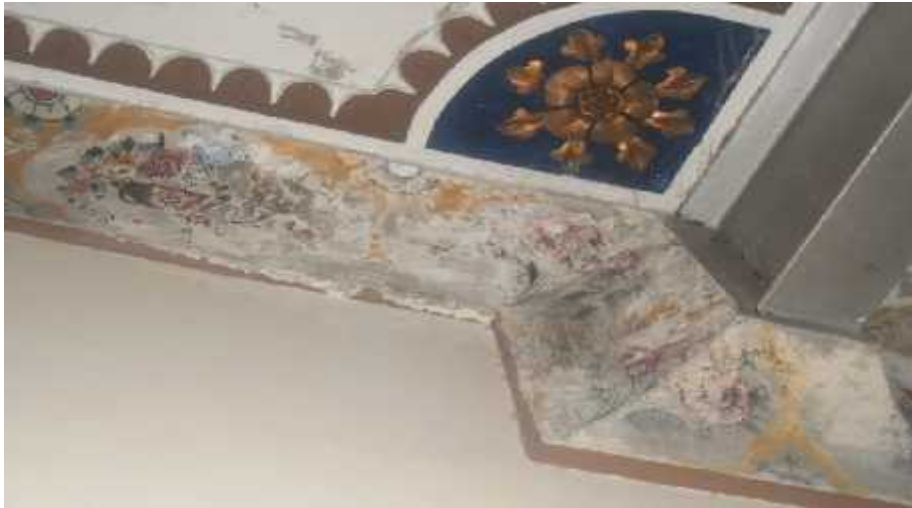
Figure 21 - Decayed painting on the beam of the roof of ground floor
